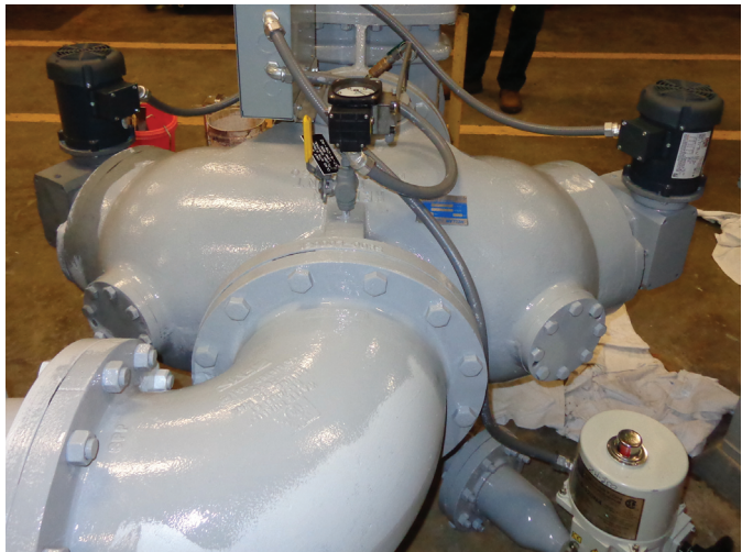
12" automatic strainer removing quagga mussels at hydroelectric plant
